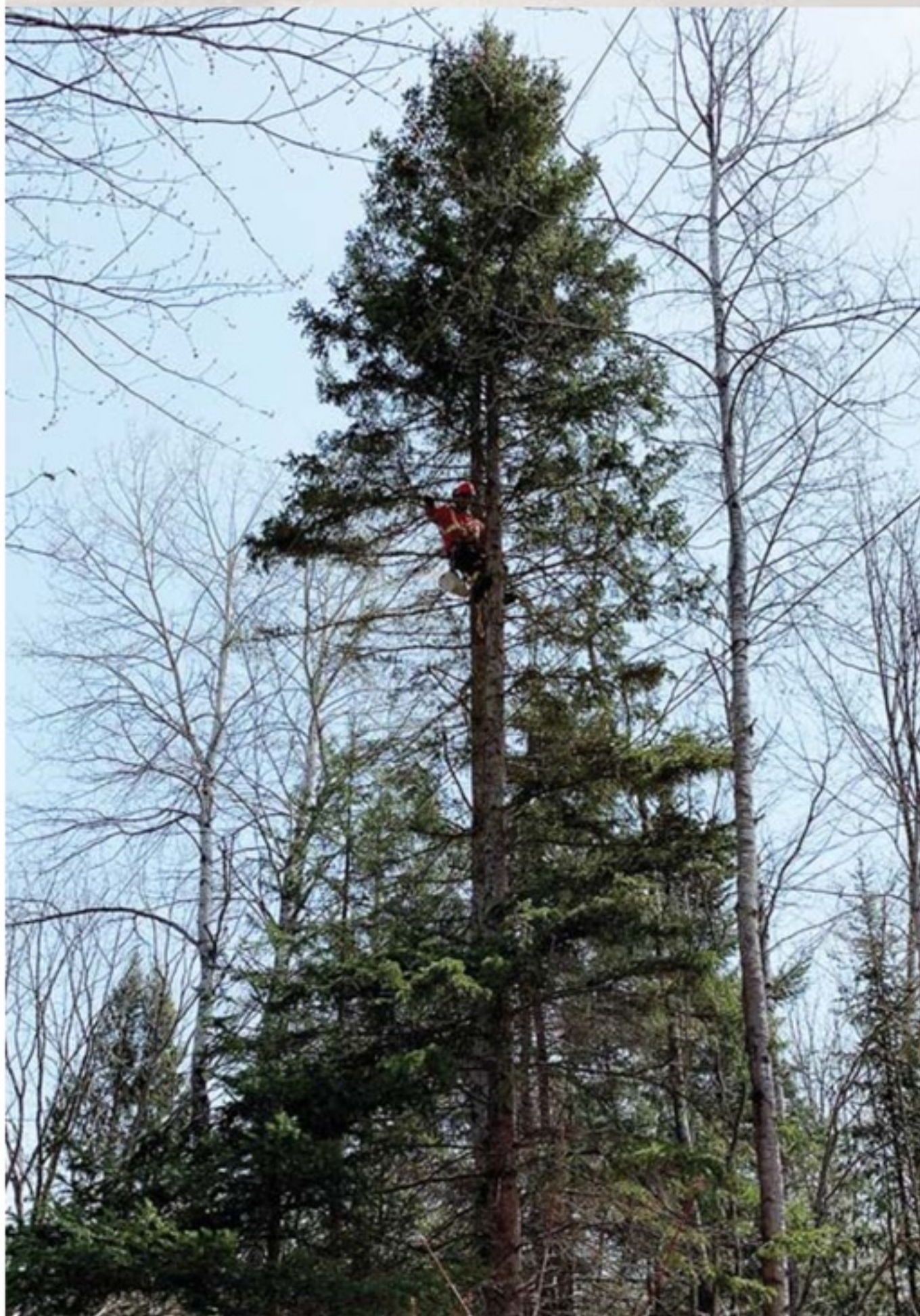
Jack Glassford, third-year apprentice, removes smaller overhanging limbs away from the line in an off-road section not accessible by truck.
