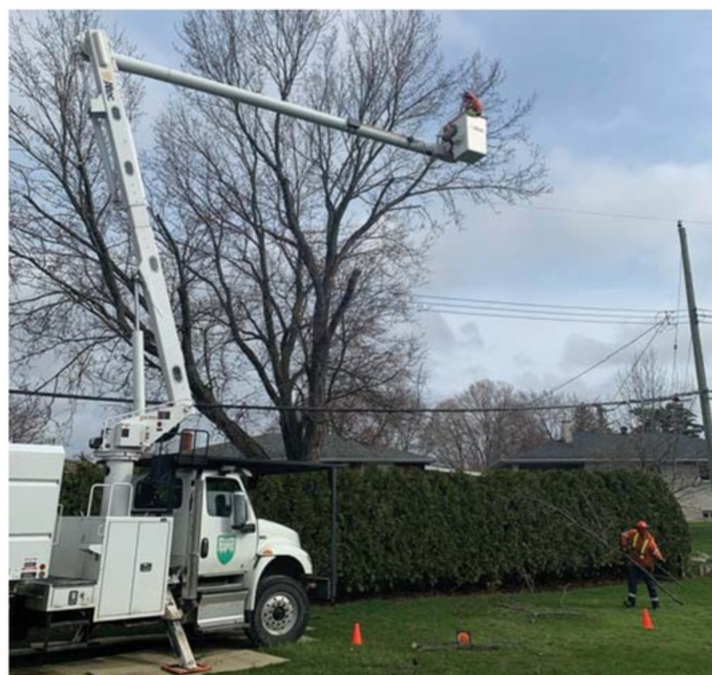
Mark Hupfl, journeyman utility arborist, clears the overhang and limbs in close proximity to make this tree safe for a local contractor to perform his work. Track mats were used in order to gain access to the backyard with the bucket truck and avoid the need for an outage and having to climb the tree.
